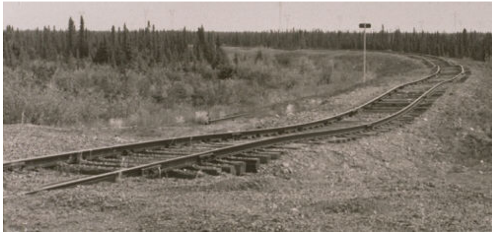
Figure 15: Ground subsidence due to thawing permafrost beneath railway tracks at Gillam, Manitoba, Canada.
