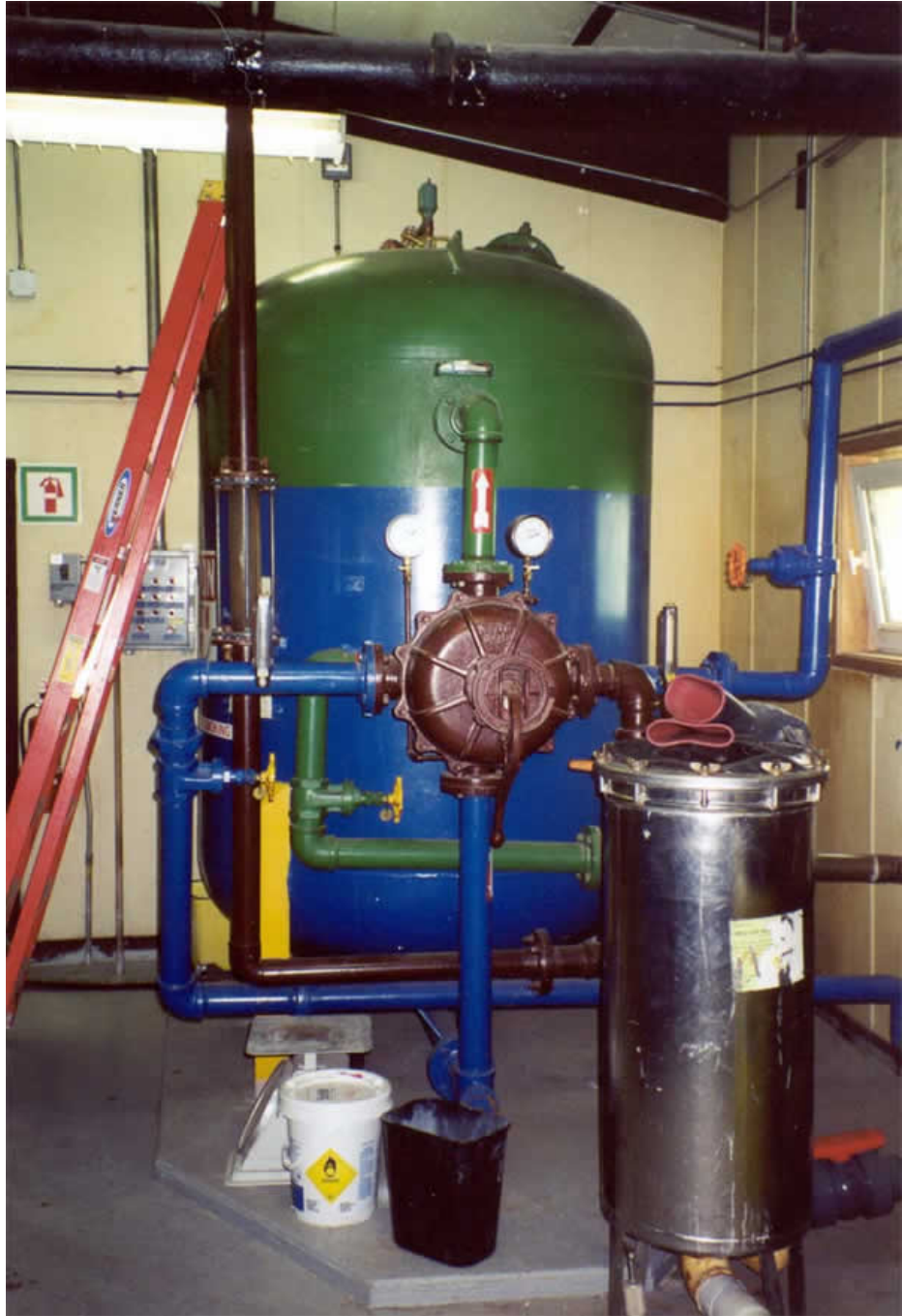
Fig. 6.4 In this figure, the green and blue steel tank in the background is a granular media pressure filter. The filter stands approximately 6 feet (2 metres) tall and is approximately 3 feet (1 metre) in diameter. In the foreground is a bag filter. Inside the stainless steel canister is a bag, much like the bag in a vacuum cleaner. The system shown is in the Arctic community of Nuiqsut in Alaska.
