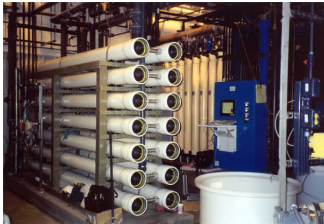
Fig. 6.5 The white tubes shown on the left are nanofilter pressure vessels. Inside the 20 plus-foot long vessels are membranes that separate dissolved contaminants from water. The tan-coloured columns on the right are pressure vessels containing microfilter membranes. These membranes remove colloidal matter from the water. Untreated water first passes through the microfilter and then through the nanofilter for complete treatment. The system shown is in the Arctic community of Nuiqsut, Alaska.
