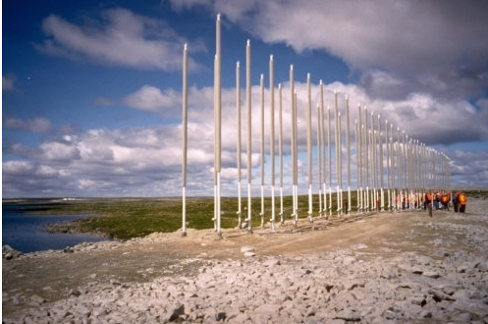
Figure 4. Thermosyphons at Lac de Gras, Northwest Territories. Source: Permafrost Regional Studies, Natural Resources Canada.
